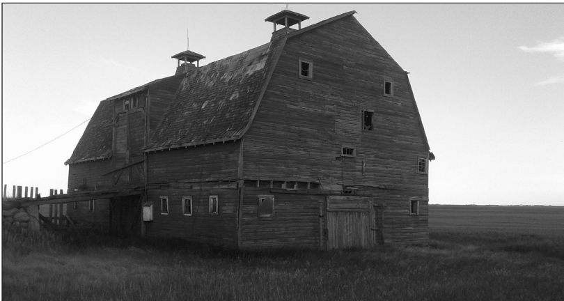
Between Marriott and Valley Centre (I think). Deceiving looks, long unused but solid on the inside. Boxstalls still need to be forked out.
